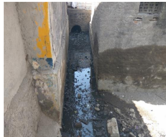
Fig.4 Sewage water Disposal
