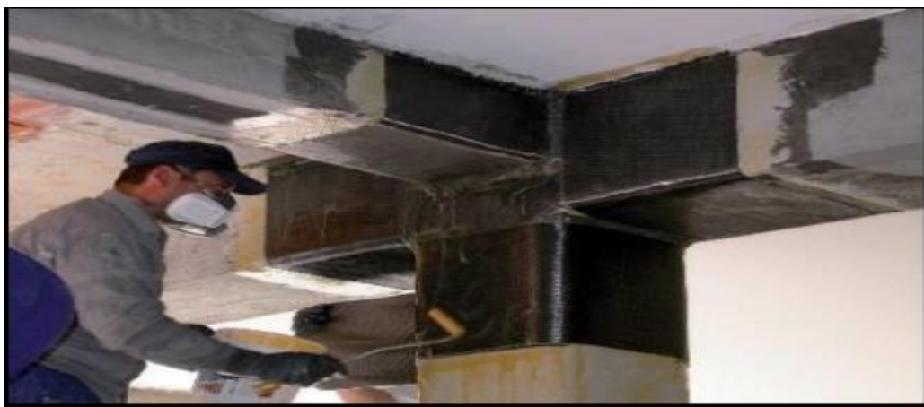
Fig.5 Fibre wrapped technique for improving load carrying capacity of beam and column
